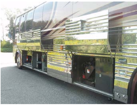
Storage bay, electrical and generator radiator bay, generator and water bay
