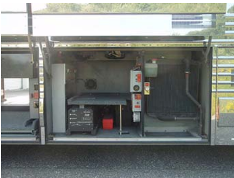
12V fuse panel, inverters, generator starting battery, generator radiator
