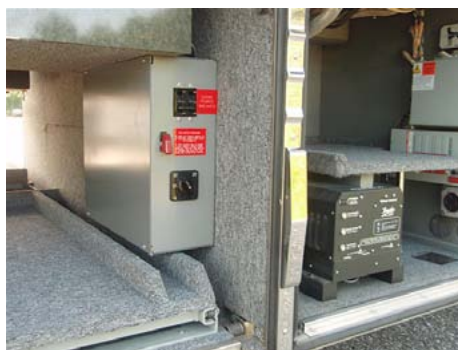
Shore power breaker and source selector switch, inverters
