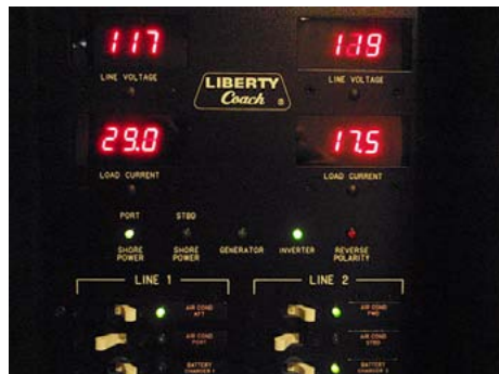
Electrical control panel
