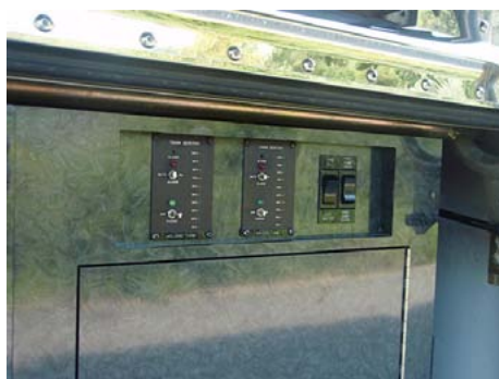
External water bay monitors and controls
