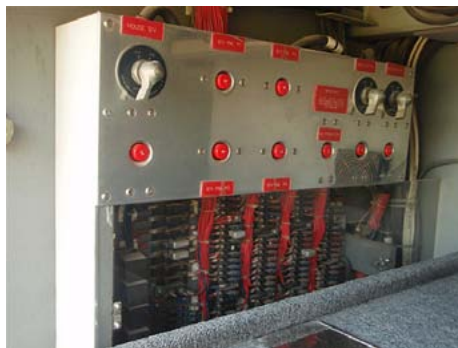
12V fuse and control area
